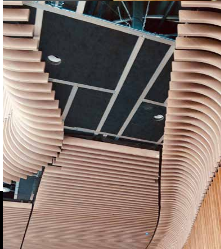
Cross-piece wood grille ceilings, walls and soffits follow lines and curves in all directions, shown here during their installation.
